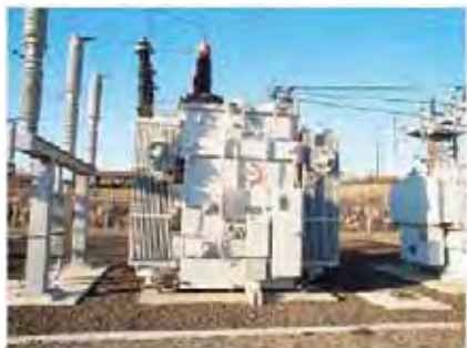
Switch Gear – Pot Heads – Corona – Leak detection
