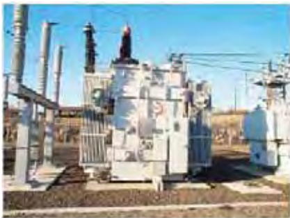
Switch Gear – Pot Heads – Corona – Leak detection
