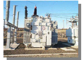
Arcing, Sparking, Corona Detection
