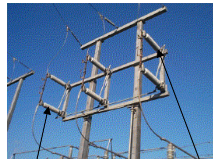
Arcing – Sparking – Tracking Corona
